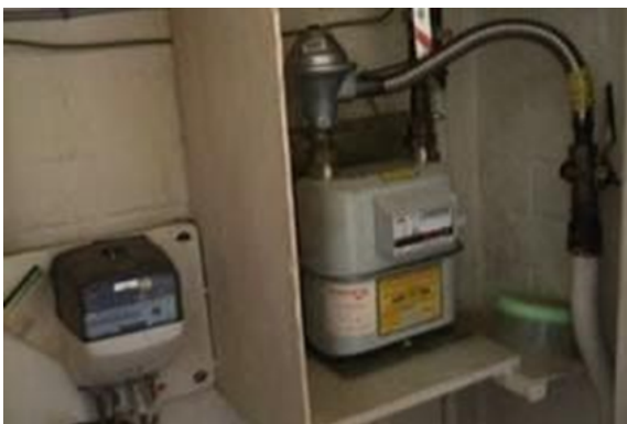
Asbestos panelling around a gas meter
