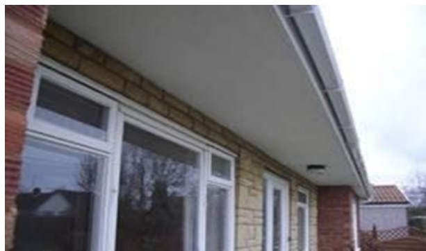
Pieces of Asbestos Insulating Board (AIB)
