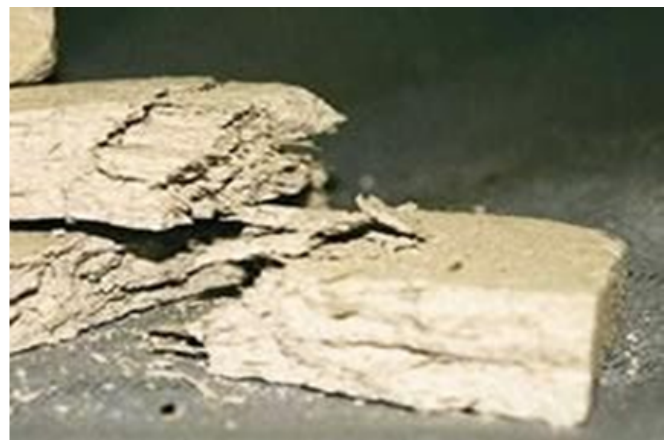
Pieces of Asbestos Insulating Board (AIB)
