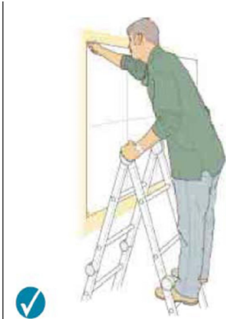
Correct – two clear rungs. Don't work any higher up this type of stepladder.
