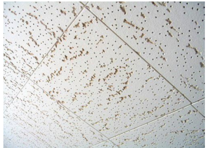
Asbestos containing ceiling tiles
