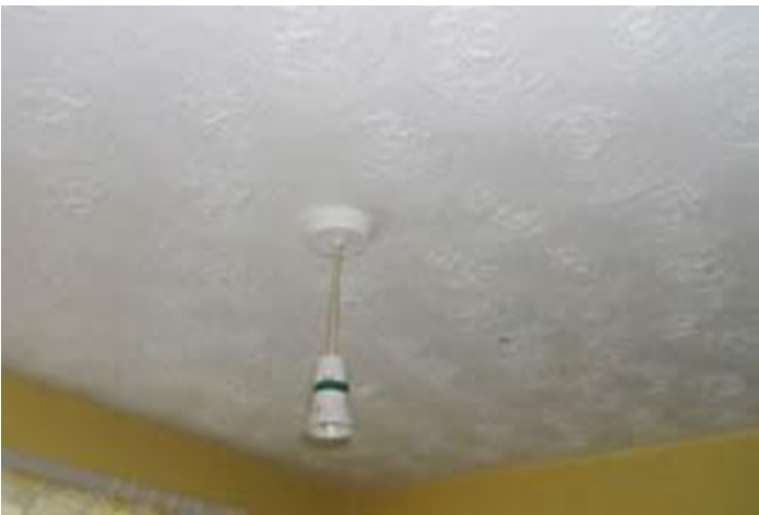
Asbestos textured coating
