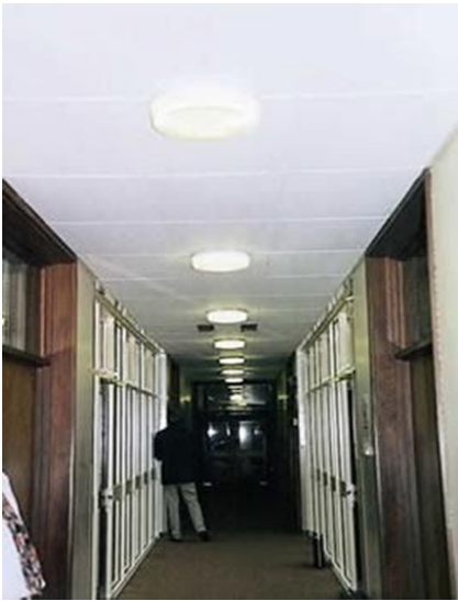
Suspended Asbestos Insulating Board tiles in a corridor
