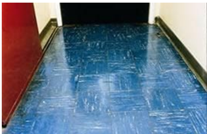
Asbestos containing floor tiles in a corridor
